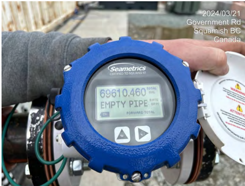
Photo 4: 01:38 PM, 03/21/24 (Flow Meter at the end of discharging)
