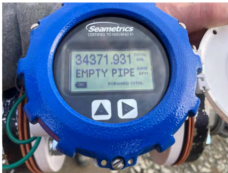
Photo 3: 09:26 AM, 03/21/24 (Flow Meter at the start of discharging)
