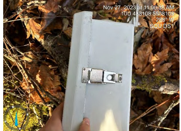
Photo 8. Location: Squamish River SQU DS1 View: West Caption: Lock cut on remaining telemetry unit cover.
