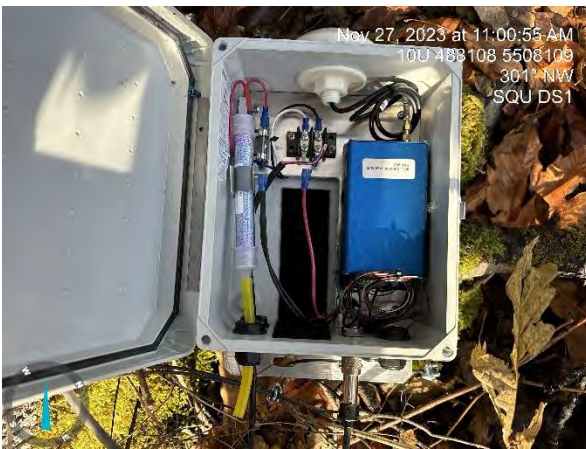
Photo 9. Location: Squamish River SQU DS1 View: Northwest Caption: Battery stolen from within remaining telemetry unit.
