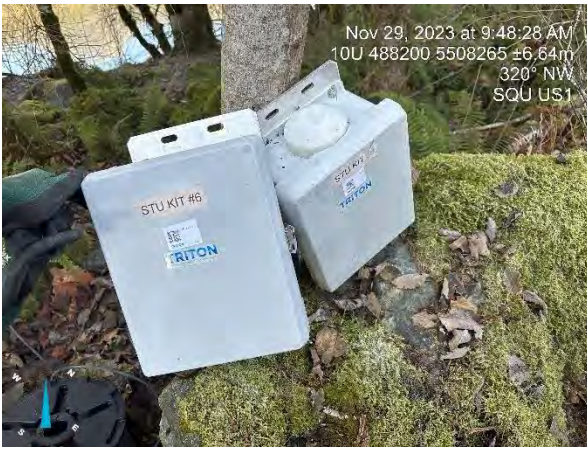
Photo 3. Location: Squamish River SQU US1 View: Northwest Caption: Telemetry and battery unit still in place and untampered with after theft of solar panel (cables securing units to tree were removed by Triton crew prior to the picture being taken).
