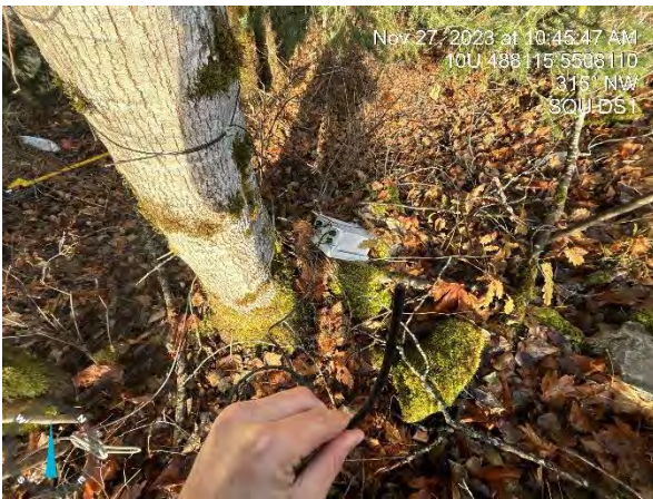
Photo 5. Location: Squamish River SQU DS1 View: Northwest Caption: Cable cut between stolen unit and remaining unit.
