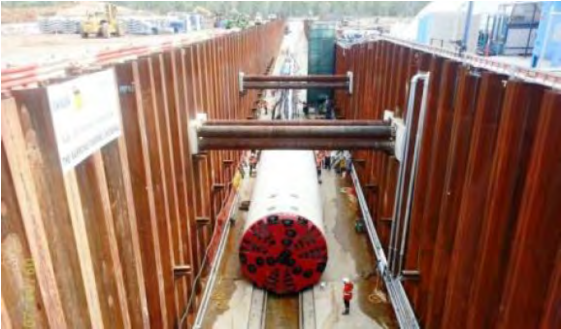
Figure 7. TBM Launch in Decline Structure with Steel Sheet Pile Walls, Steel Strut Support and Concrete Base Slab; Narrows Crossing, Australia
