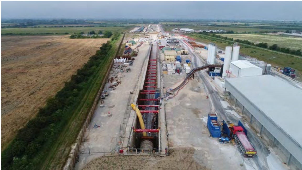
Figure 6. Plan View of Decline Structure for TBM Launch and Pipeline Installation; Humber River, United Kingdom
