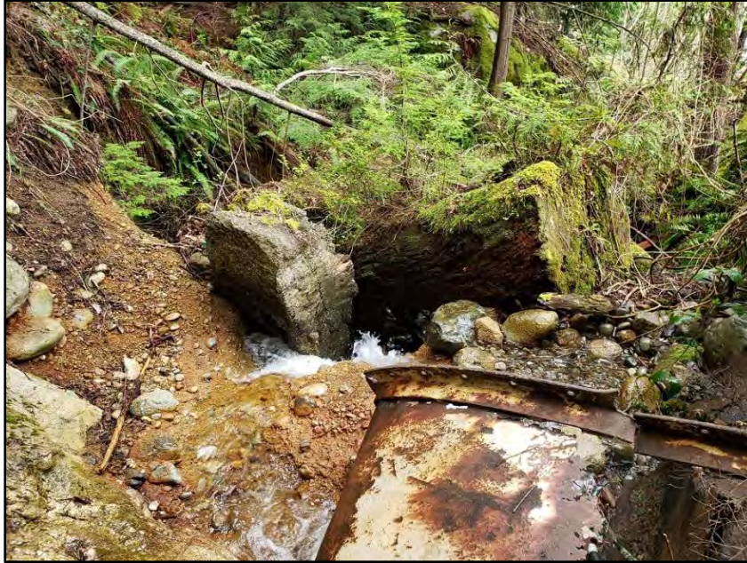
Photo 5. View downstream approximately 20 m upstream of the proposed discharge location, showing bank instability and metal debris/boulders in the watercourse. (April 17, 2019).
