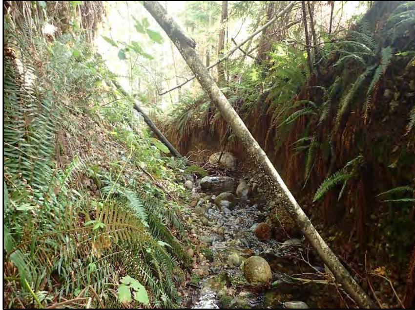
Photo 3. View downstream of bank/fill erosion, approximately 40 m upstream of the proposed discharge. (October 4, 2019).
